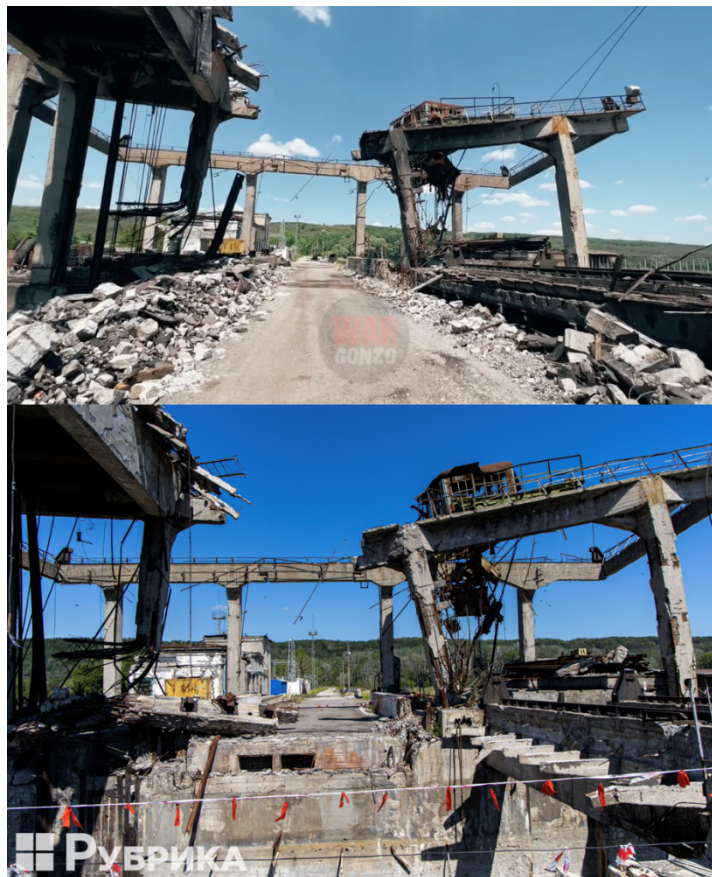
Figure 12: Oskil Dam road span above the first gate in various stages of destruction. From top to bottom: Published on May 23, 2022; published on August 31, 2023.
