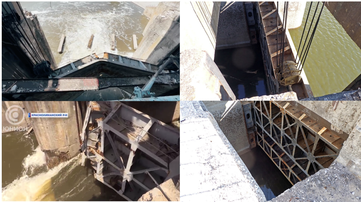
Figure 10 Left: Screenshot of the destroyed Oskil Dam gate broadcast on the DPR television station UNION. Image published on May 25, 2022. Right: Photograph of an alleged repaired Oskil Dam gate published by the DPR Ministry of Emergency Services. Published on June 7, 2022.
